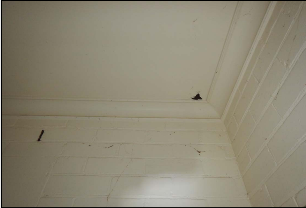
Photo 21: Building 13 - Ceiling sheet outside upper floor bathroom
