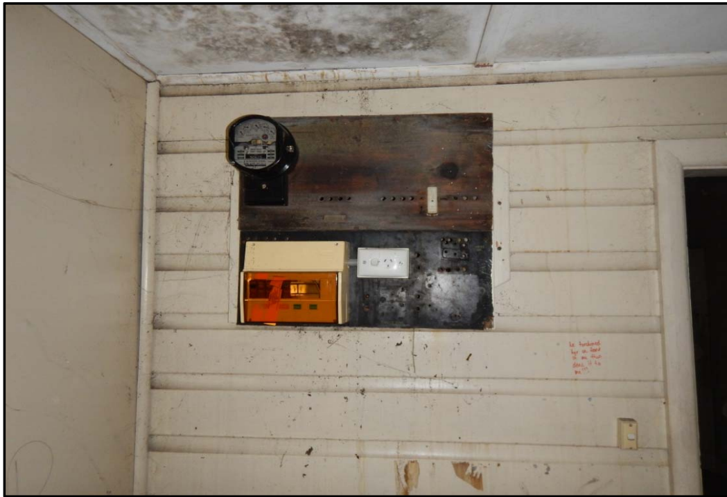
Photo 9: Building 11 - Electrical Board
