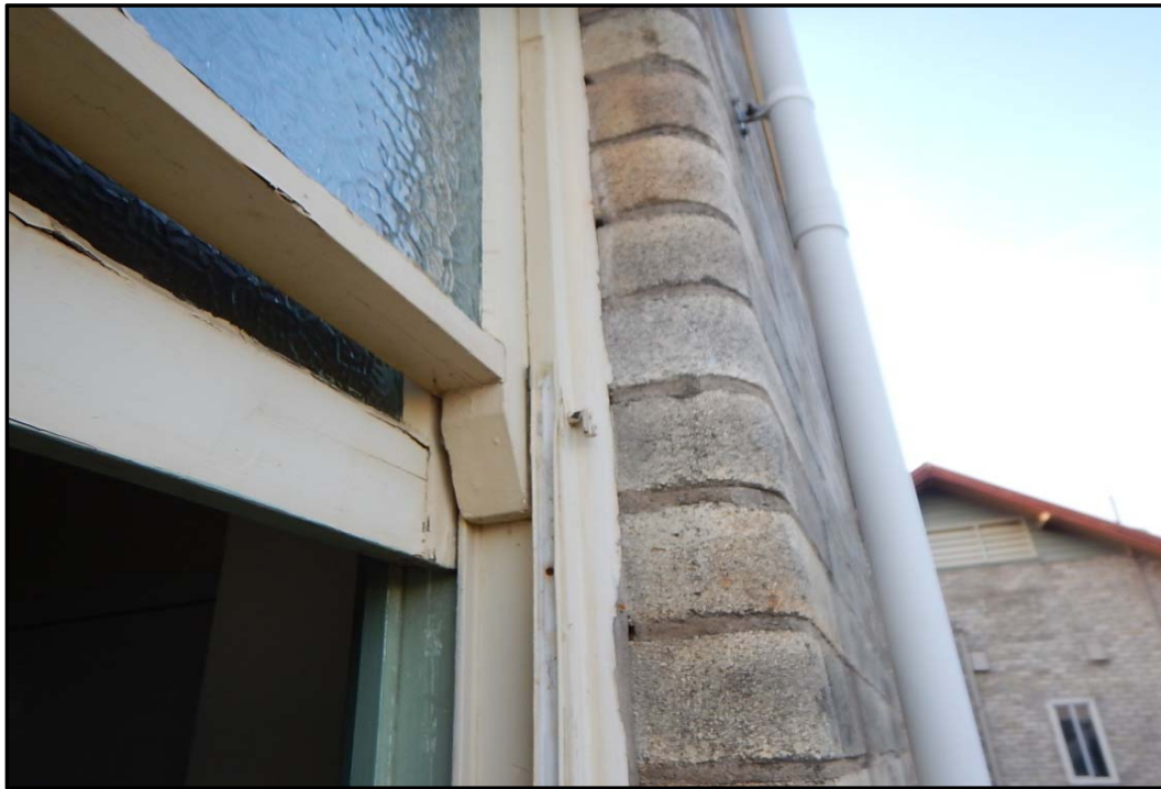
Photo 25: Building 13 - Lt yellow/cream exterior paint upper storey bathroom
