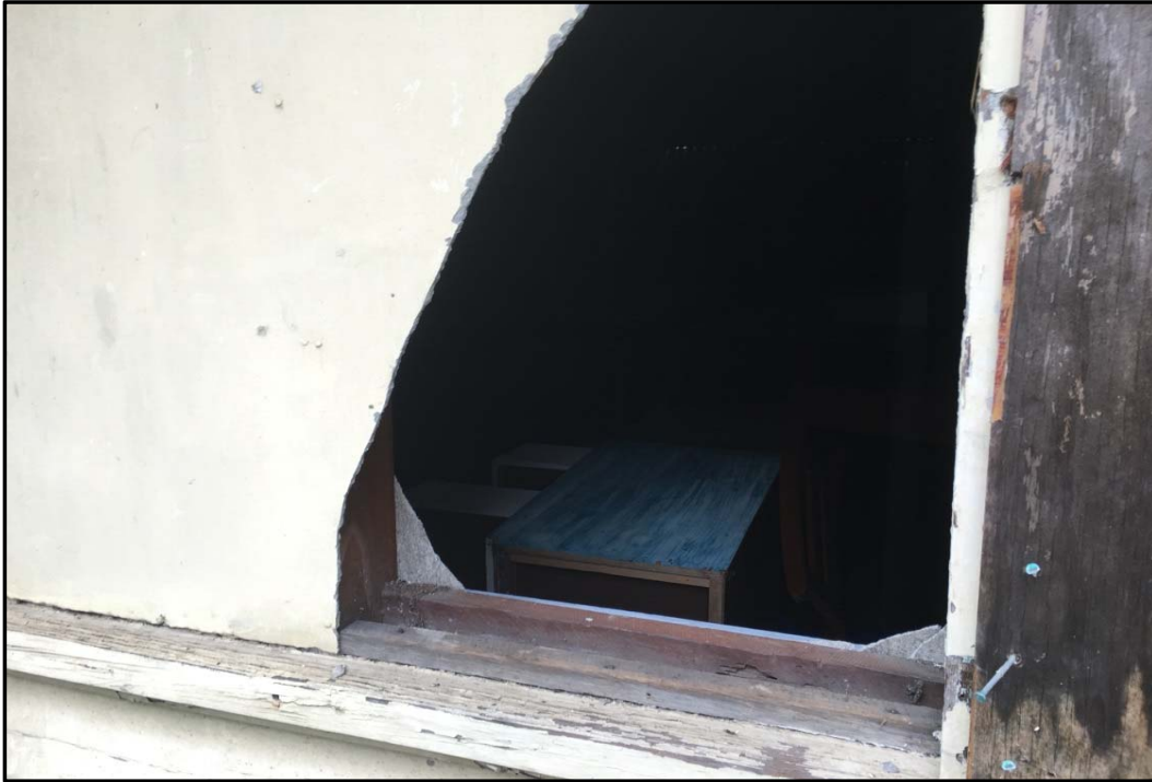
Photo 30: Building 14 - Damaged external and internal wall linings
