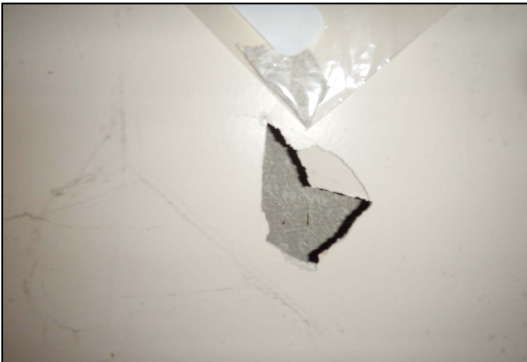
Photo 4: Building 11 - Wall sheathing in sunroom
