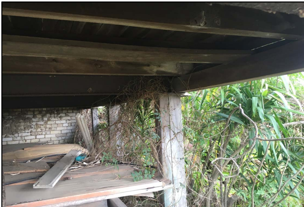
Photo 35: Building 14 - Subfloor zone with assumed lead damp proof course over brick footings
