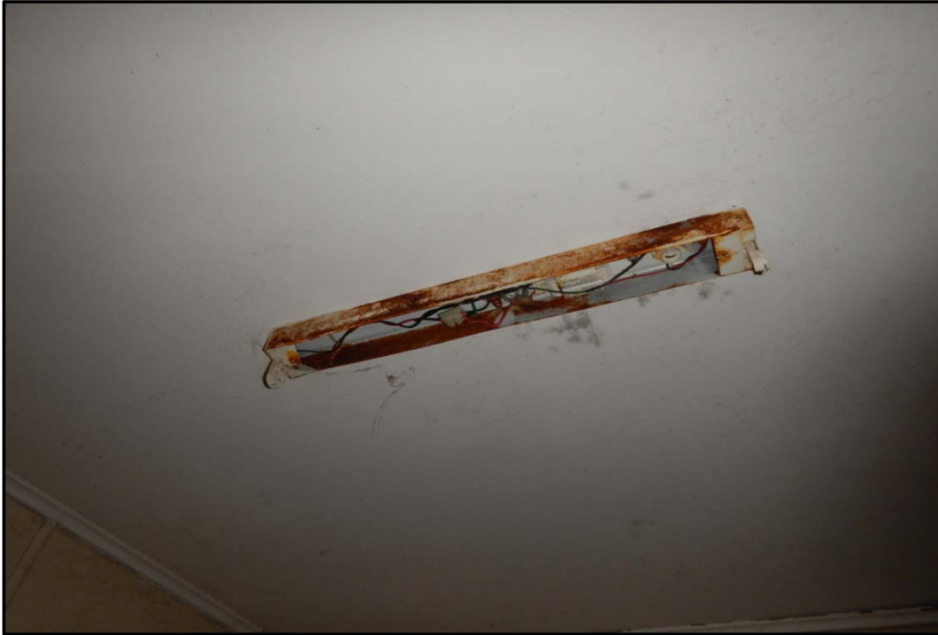
Photo 13: Buildings 10 and 11 - Fluorescent lighting
