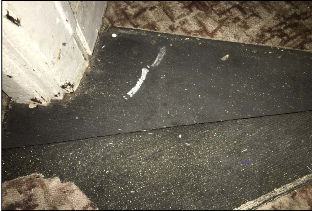
Photo 36: Building 14 - Carpet underlay assumed to comprise SMF
