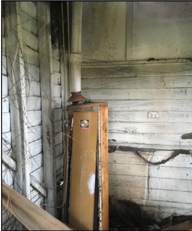
Photo 34: Building 14 - Hot water system with cement flue assumed to comprise ACM
