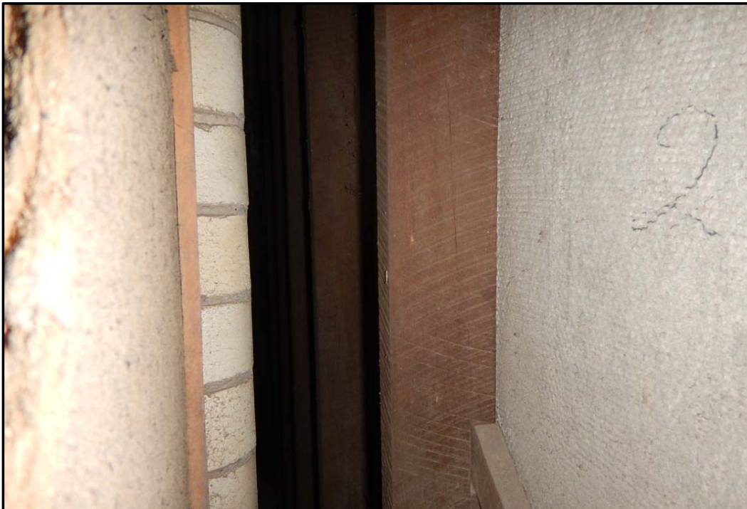
Photo 22: Building 13 - Asbestos common wall between Buildings 13 and 14
