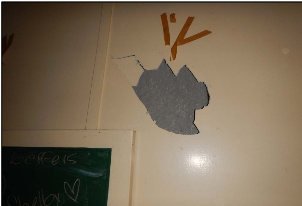
Photo 2: Building 10 - wall sheeting in classroom above picture rail
