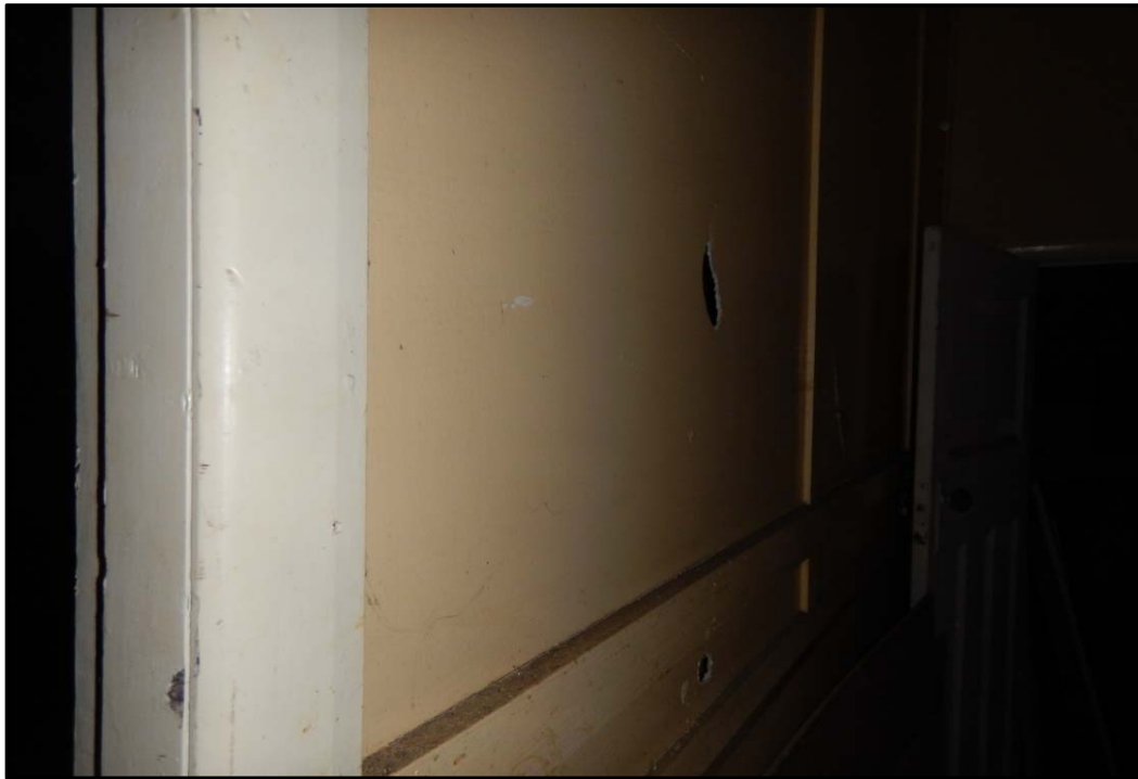
Photo 1: Building 10 - Wall sheeting above picture rail in hall (all rooms)
