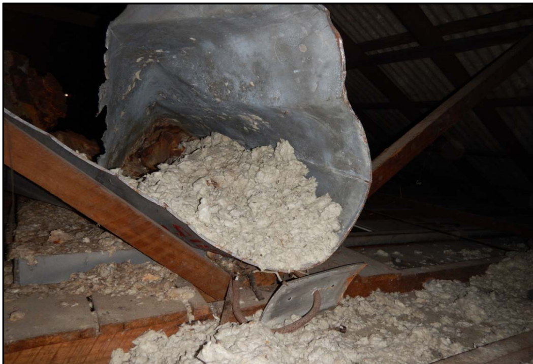
Photo 10: Building 11 - Fibrous material in roof space
