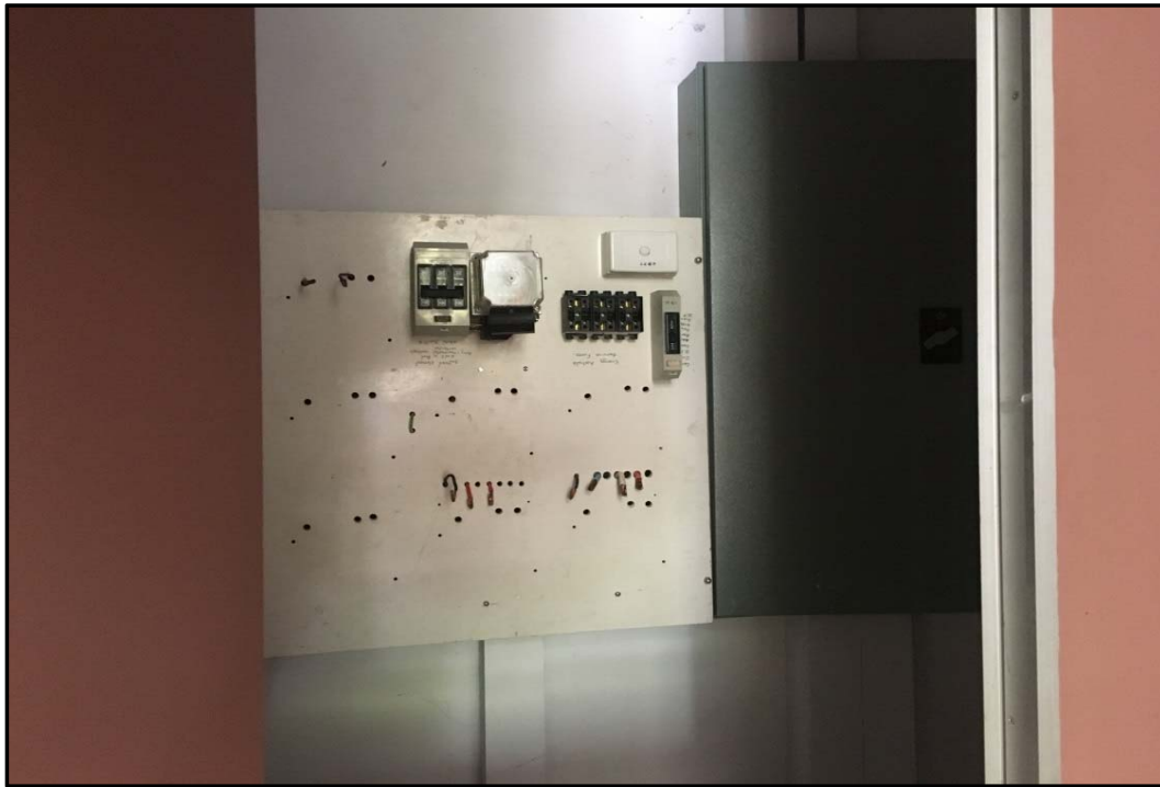
Photo 18: Electrical Distribution Board, First Floor
