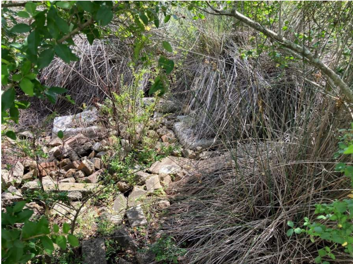
Photograph 11: Building rubble placed in central dam as scour protection (as advised by owner) Lot 1308.
