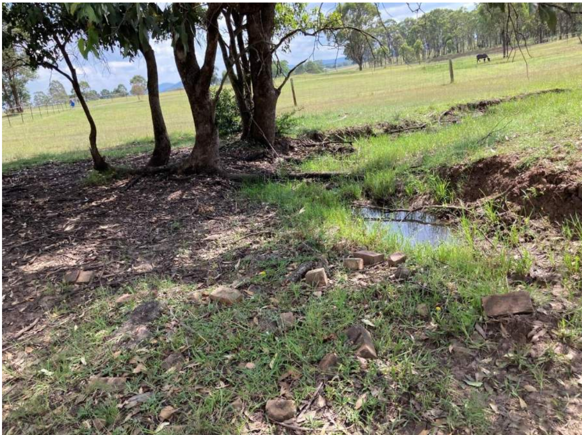
Photograph 12: Building rubble placed in drainage line as scour protection (as advised by owner) Lot 1308.
