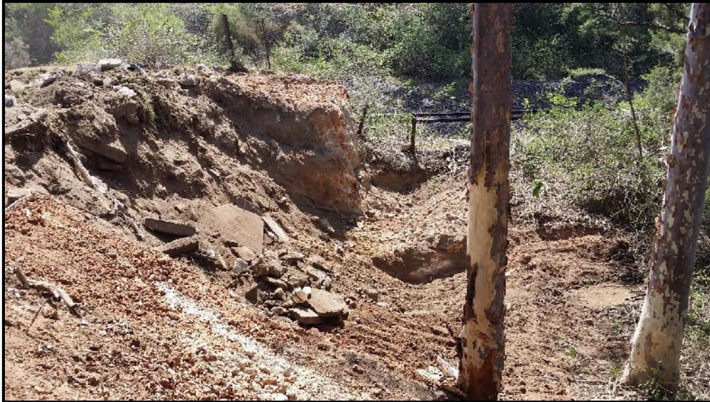
Print 3 Excavation progress of the northern end of the Western Fill Zone.
