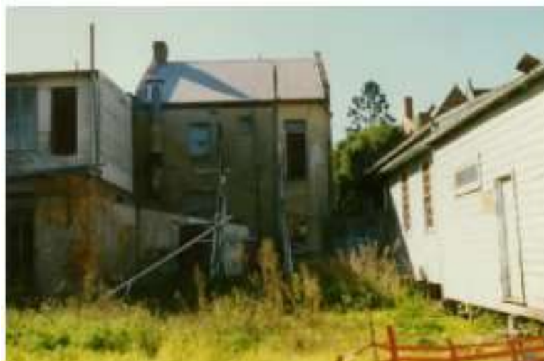
FIGURE 2.25 - VIEW OF REAR EXTENSIONS AT 271 HIGH STREET PRIOR TO DEMOLITION (AT LEFT).
