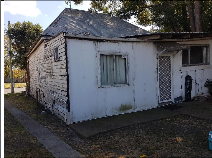
Photo 11 East-Southeast to West-Northwest perspective; dwelling at 11 Louth Park Rd. Dwelling tenanted and in moderate condition. Potential ACM on dwelling.
