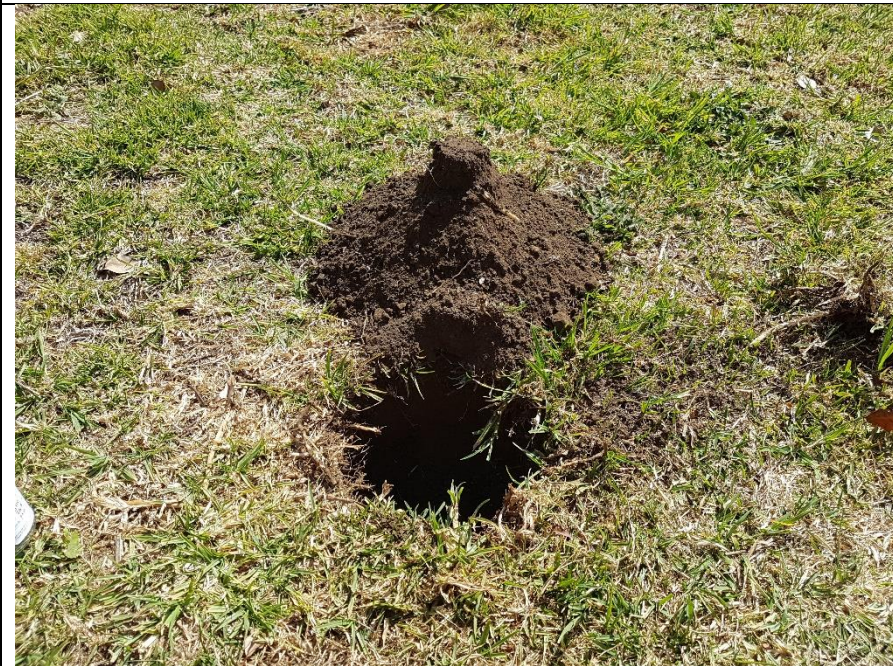
Photo 8 Southeast to Northwest perspective; borehole BH07 at rear yard of 5 Louth Park Rd.
