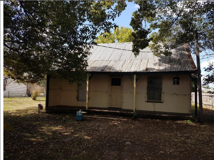
Photo 3 West to East perspective; dwelling at 9 Louth Park Rd. Unoccupied and in poor condition. Potential ACM on dwelling & debris at front of dwelling.
