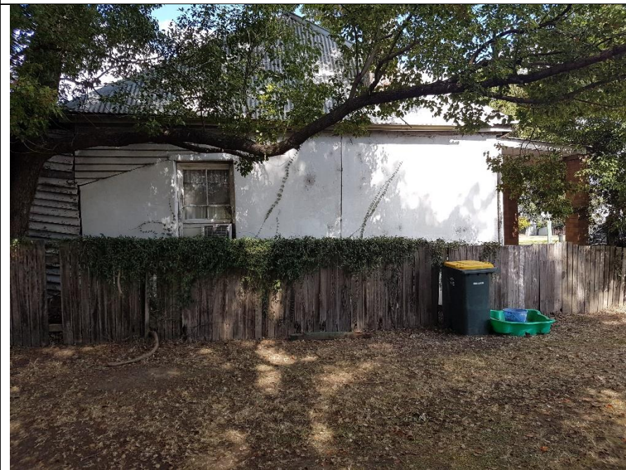
Photo 4 North to South perspective; north wall of dwelling at 11 Louth Park Rd. Tenanted and in moderate condition. Potential ACM on dwelling.
