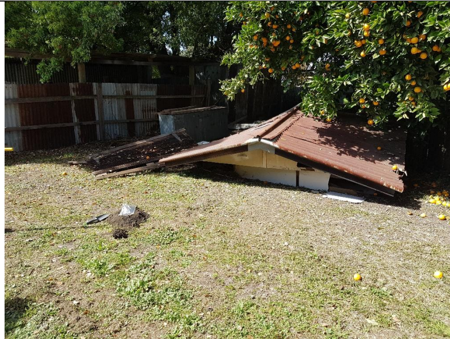
Photo 5 West to East perspective; shed at rear of 9 Louth Park Rd. Collapsed and in very poor condition. Potential ACM debris.
