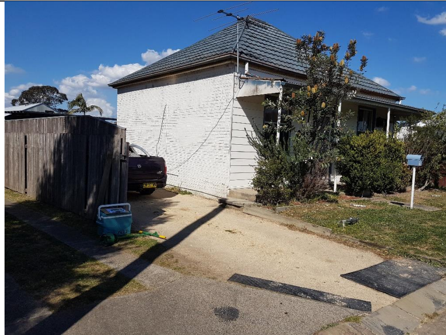
Photo 13 Northwest to Southeast perspective; dwelling at 13 Louth Park Rd. Dwelling tenanted and in good condition. Potential ACM on dwelling.
