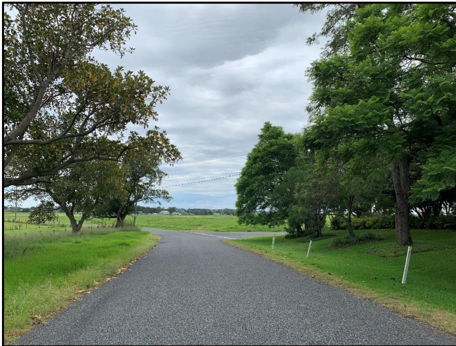
Photo 1 – View looking north along Swan Street showing typical cross section and intersection with Brisbanefield Road
