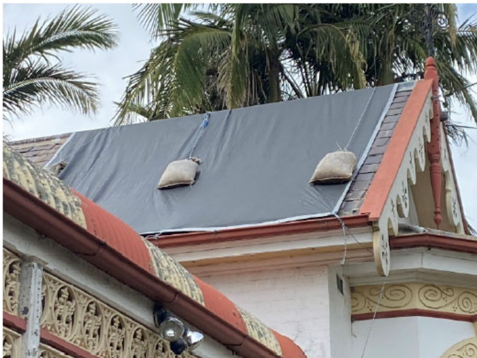
Figure 2 – Current Roof Condition
