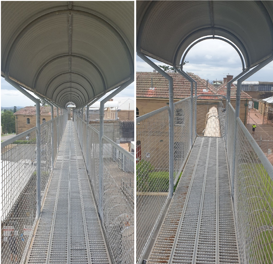
Detail views of typical walkways (Gantry Walkway 3 at left and Gantry Walkway 1 at right)
