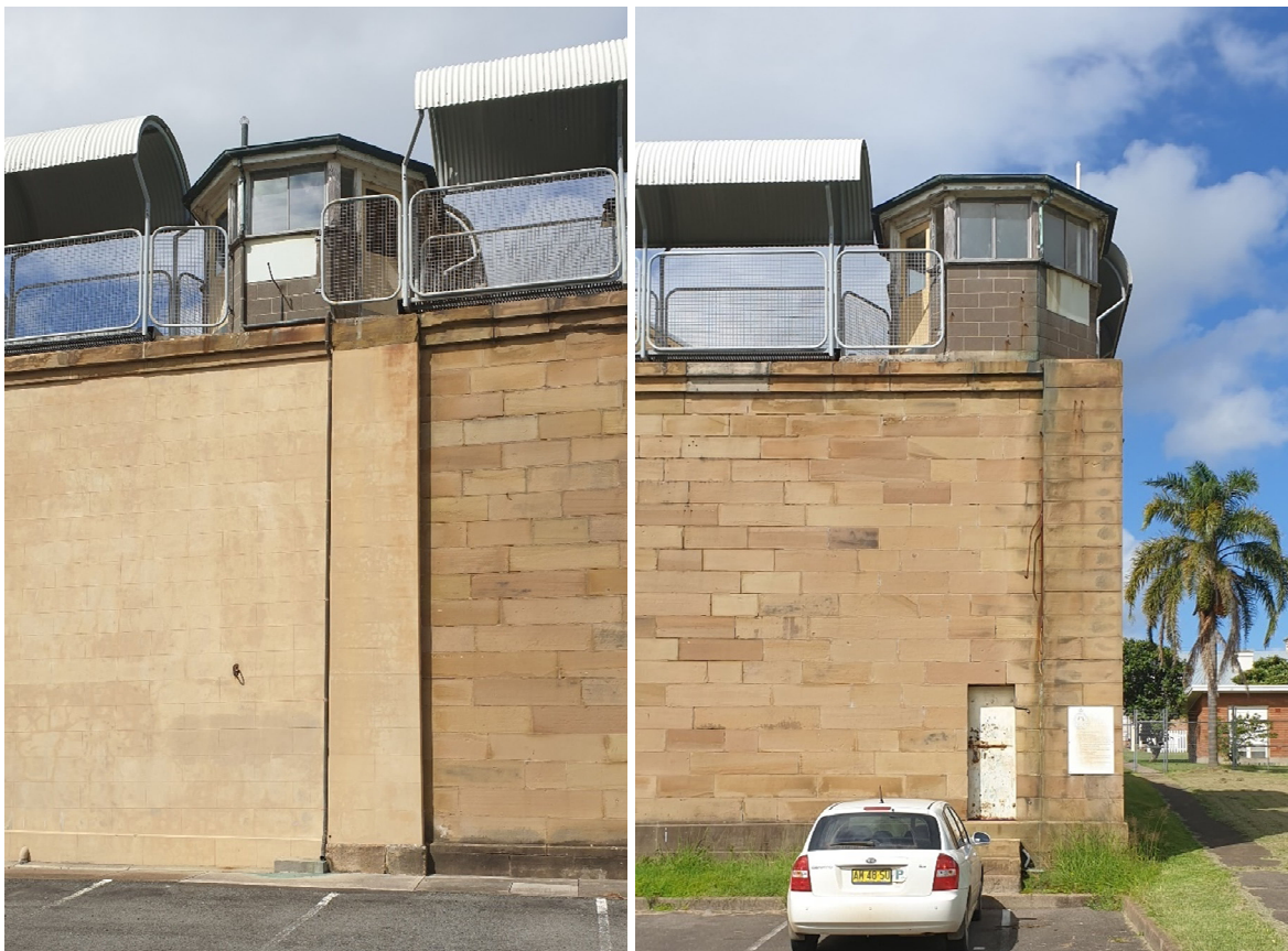
Stormwater downpipes at Towers 1 and 6 (downpipe largely missing at Tower 6 on right)
