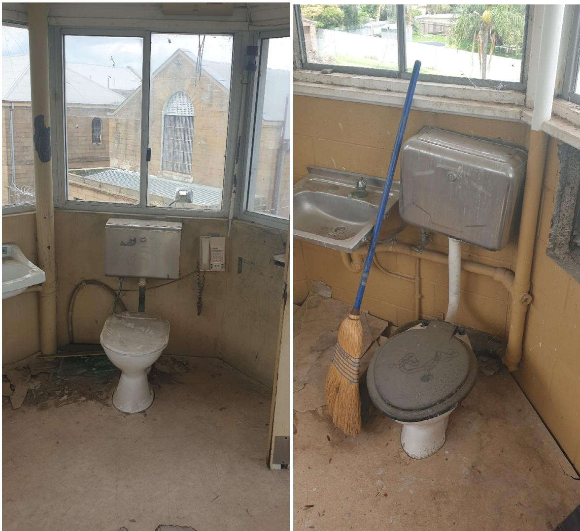
Existing toilet and handbasins in Tower 1 (left) will be lost and those inside Tower 6 (right) will be retained for interpretation
