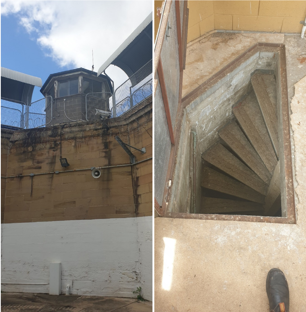
Tower 6 viewed from within former prison yard looking south and access hatch inside the tower
