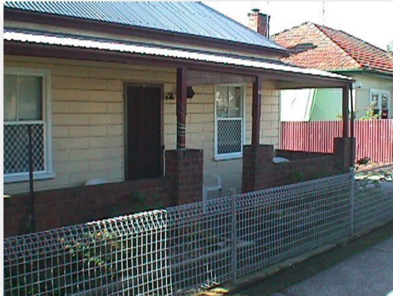
This verandah brick wall could be removed and timber posts reinstated to return the cottage to its original design and improve its appearance
