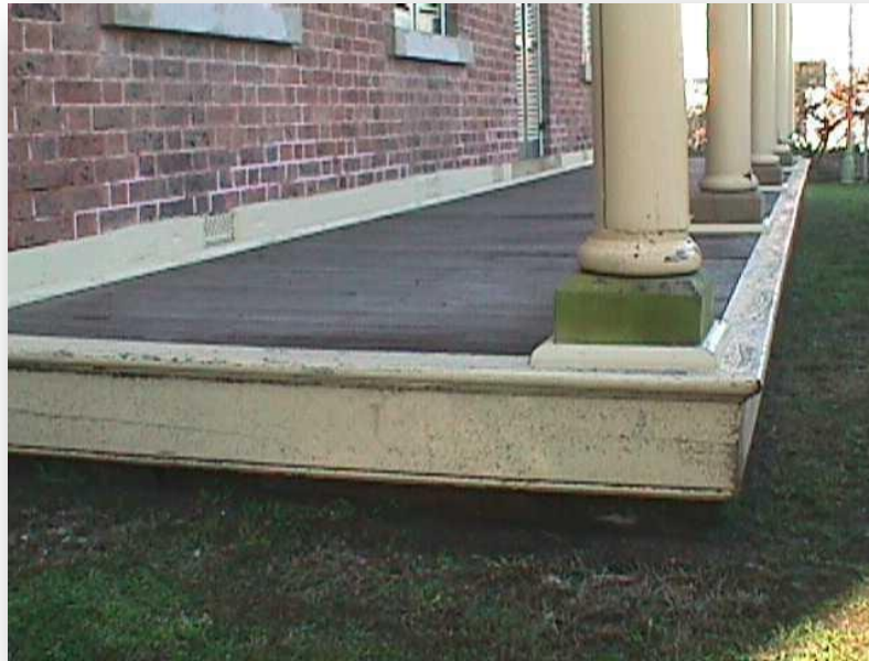
Wooden items need regular maintenance and should be inspected every six months
