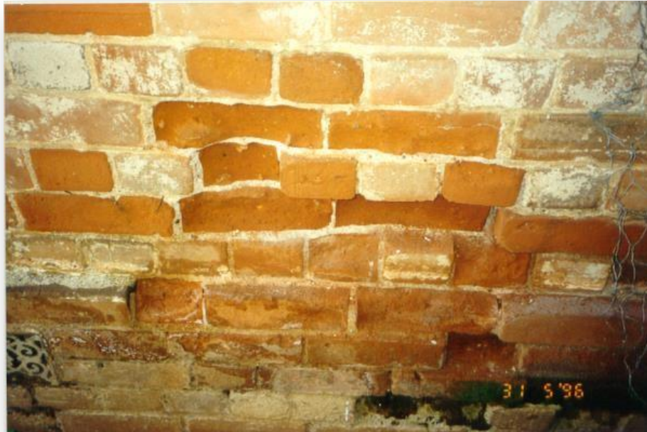
Rising damp and salt attack can lead to serious deterioration of masonry
