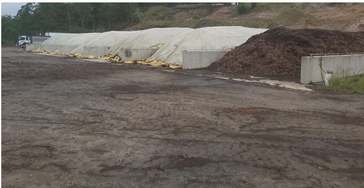
Figure 7 – Trafficable engineered clay liner adjacent to the composting bunkers showing no signs of degradation or deformation.
