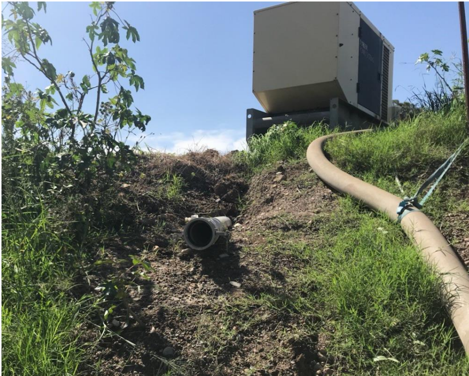
Figure 6 – Inlet of 100 mm diameter overflow pipe at Stormwater Storage Dam which directs flow to Sediment Dam 1 and 2
