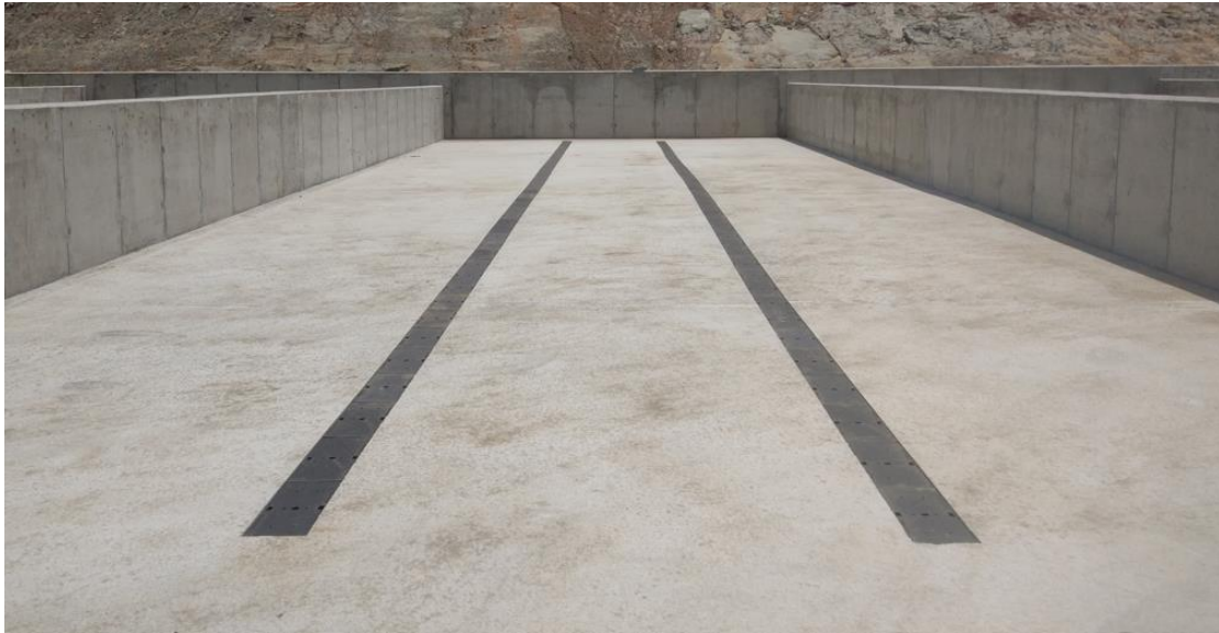
Figure 2 – Constructed concrete bunker with pair of dual purpose channels for aeration input and leachate drainage.
