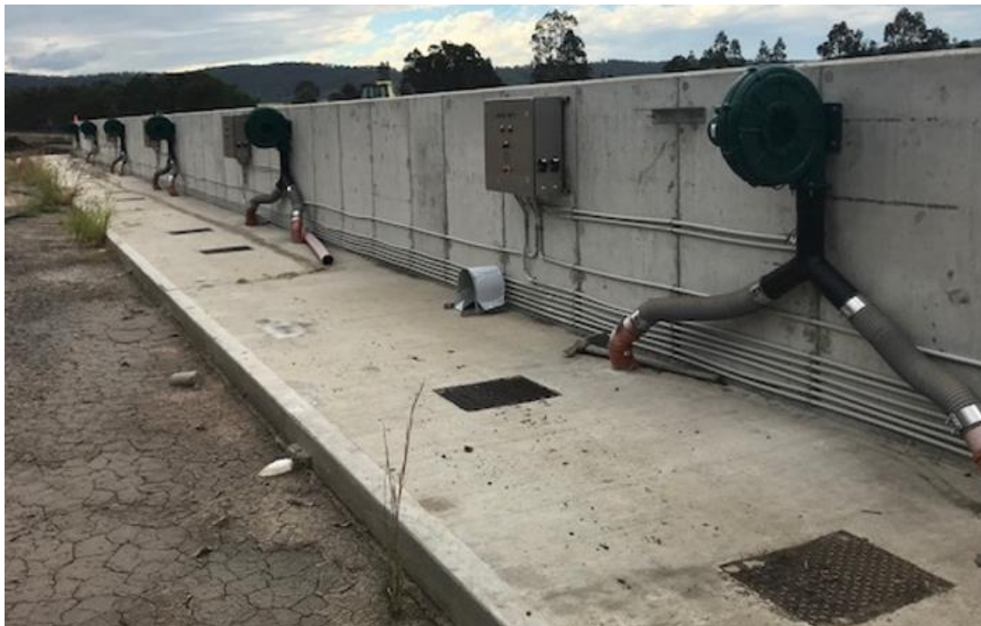
Figure 3 – Air compressors mounted at the back wall of each compost bunker and covering plates over a pair of leachate drainage sumps per bunker.
